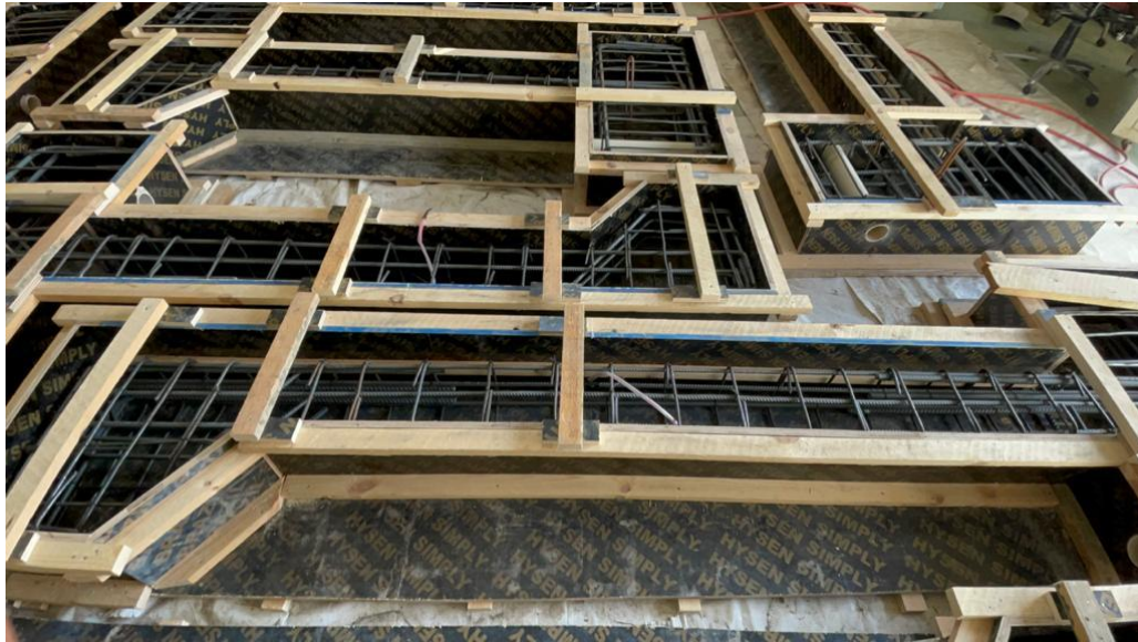
Figure 3.11 Column specimens after strengthening the formwork and adding the strain gauges ready for concrete casting
